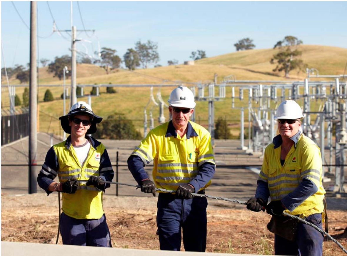
Workers splice a cable in preparation to connecting electricity to the power substation
